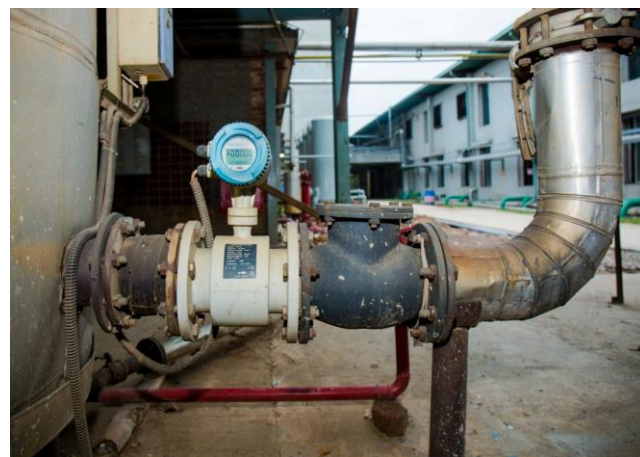
Photo: Water Flow Meter which is used for cooling water measurement
