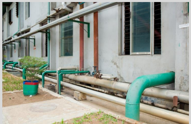
Cooling water pipeline interconnected to main header line. After this, pipeline is connected in to the main reserve tank. JM Fabrics Ltd.
