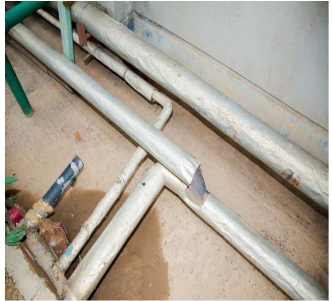
Cooling water pipeline interconnected to main header line which is shown in the image. This pipeline then after connected in to the main reserve tank. JM Fabrics Ltd.
