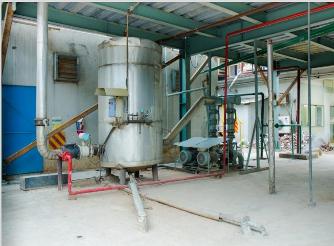
Underground water reserved tank (capacity-90,000 Ltr) and water transferring pump (capacity-15Kw) with water vessel. All these are important for water storage and supplying
