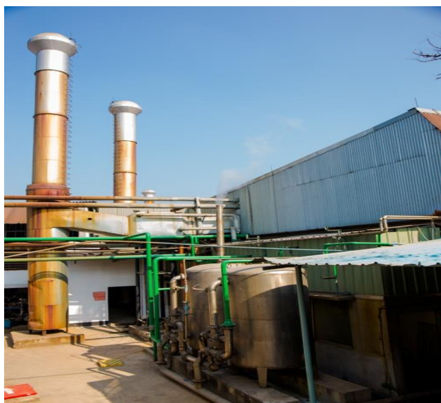
Boiler Economizer at Zaber & Zubair Fabrics Ltd.
