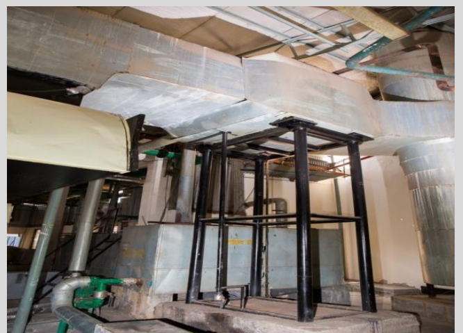
Closer look of Boiler Economisers of Zaber and Zubair Fabric Ltd.
