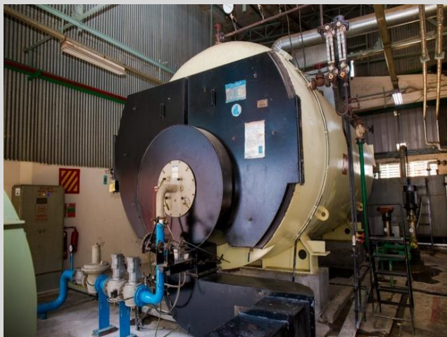
Boiler, Zaber and Zubair Fabric Ltd.
