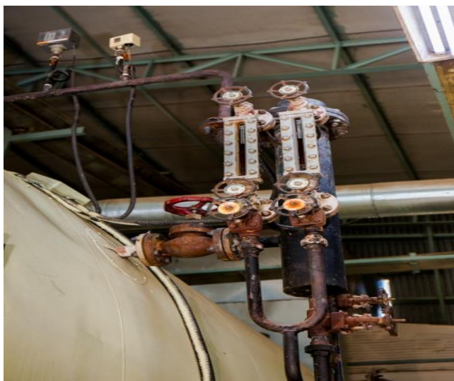
Steam pressure meter of Boiler
