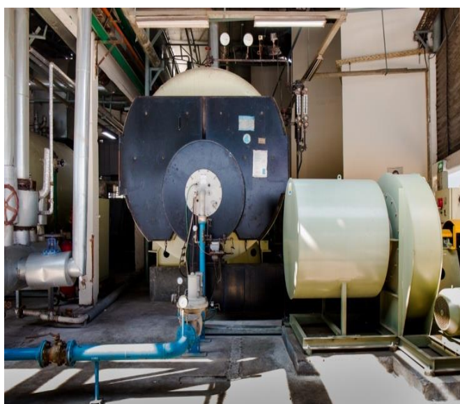
Boiler, Zaber & Zubair Fabrics Ltd.
