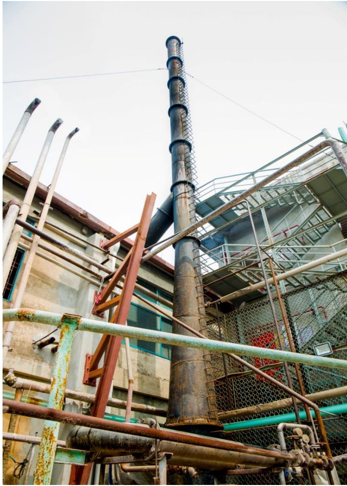
Chimney of Exhaust Gas Boiler
