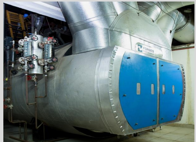
EGB Gas Boiler (3.1) at One Polar Ltd
