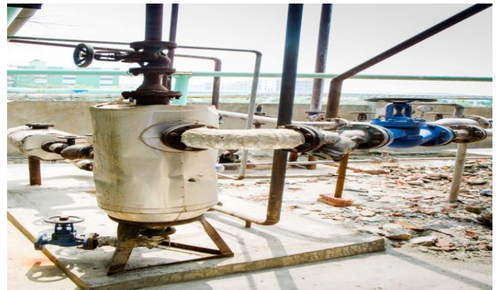
Condense Set ( Heat Exchanger)
