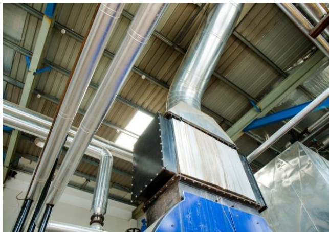
Economiser of Gas Boiler
