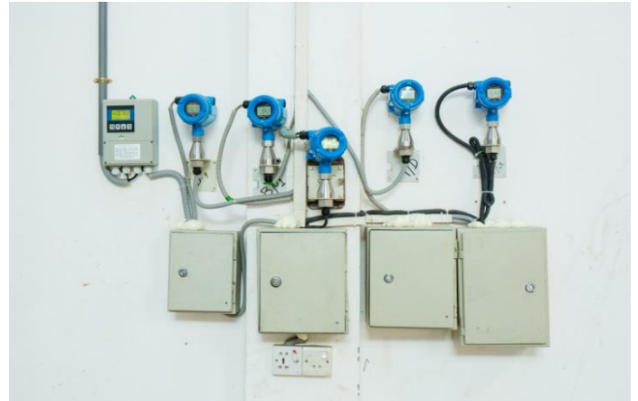
Steam Flow Meter Control Box
