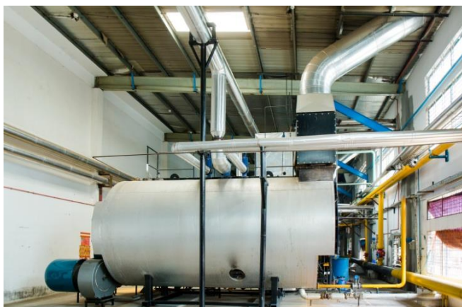
as Boiler 2 at One Polar Ltd.
