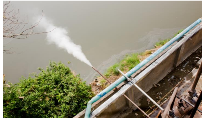
PPPP Pump Flash Steam
