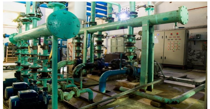
Make Up Water Pump
