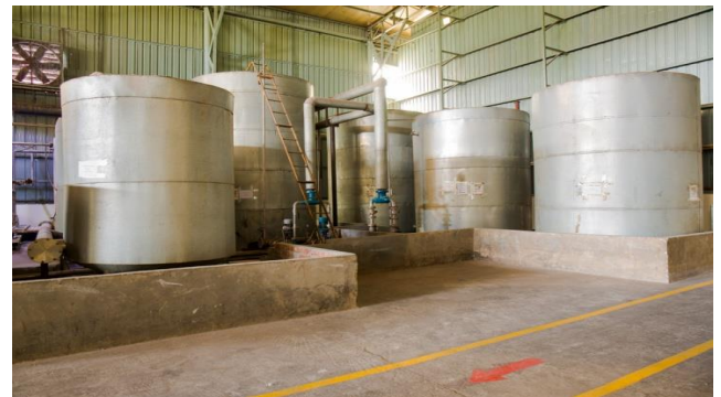
Refining Tanks of Caustic Recovery Plant (CRP) at Zaber & Zubair Ltd.
