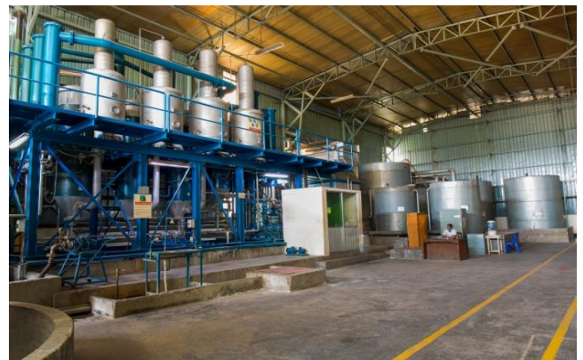
Caustic Recovery Plant (CRP) at Zaber and Zubair Fabrics LTD
