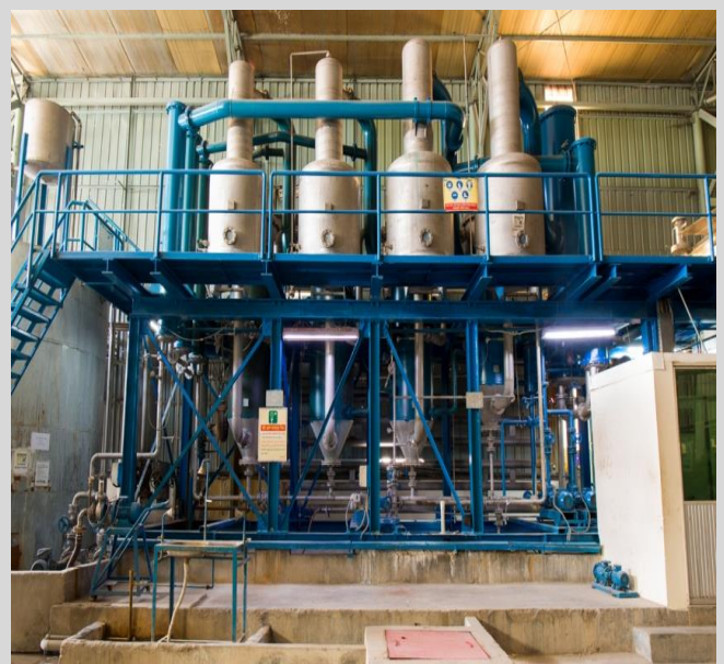
Weak Lye Tanks of CRP at Zaber & Zubair Fabrics Ltd.
