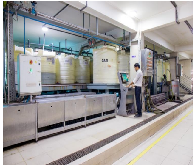
A Production Officer monitoring the Chemical dosing process at DBL Group, Gazipur
