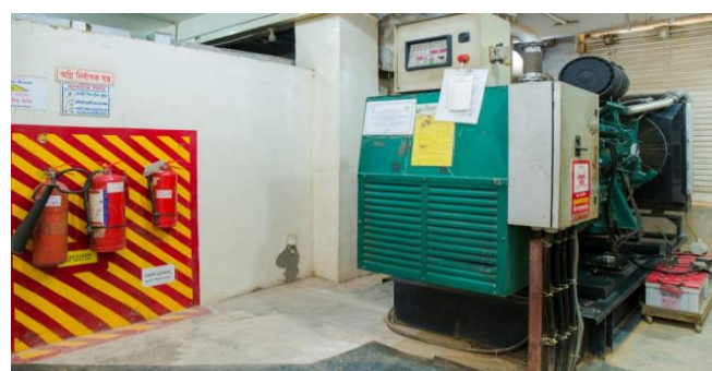
Diesel Generator Set
