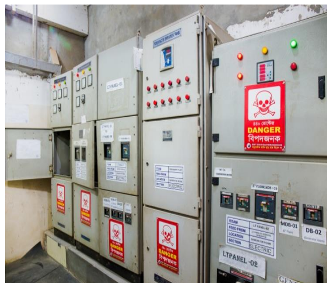
LT Panel & MDB (Main Distribution Board) Panel
