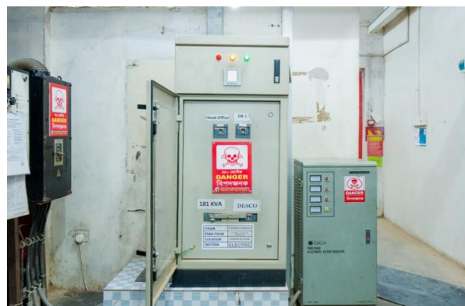
MDB & Automatic Charger / AVR Panel
