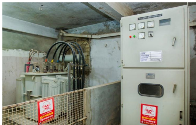
Transformer & HT Panel
